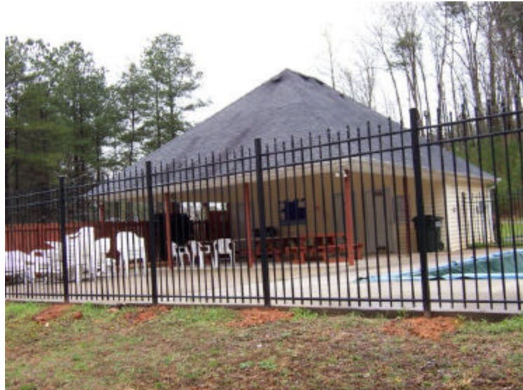
Here's how the new fence construction looked on Thursday with three sides completed.
